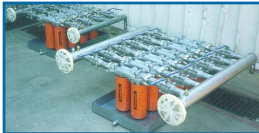
COST-EFFECTIVE DUPLEX ALTERNATIVE: In this application, the manifolds have on/off valves so that filters can be changed without shutting down the whole system.
